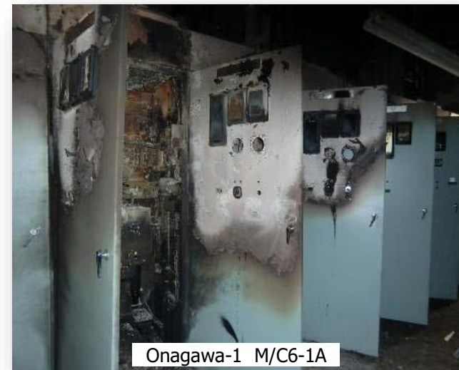
Figure Damage to metal-clad switchgears caused by the HEAF event at unit 1 of Onagawa nuclear power station ( http://warp.da.ndl.go.jp/info:ndljp/pid/10378577/www.nsr.go.jp/data/00160077.pdf )
