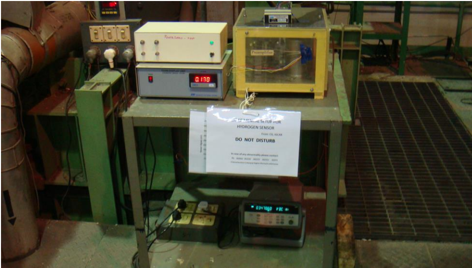
Fig. 4 Photograph showing the installation of \text{SnO}_2 sensor at the TCD outlet in the secondary sodium circuit (west) of FBTR
