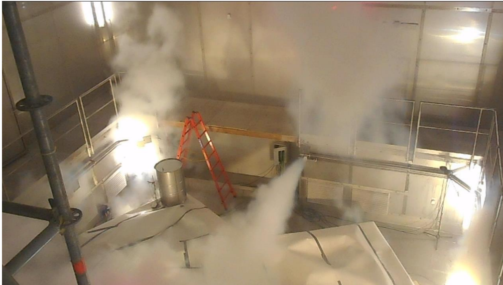
FIG. 3. First test of the fire extinguishing system using liquid argon which evaporates immediately at the outflow nozzles in the containment.
