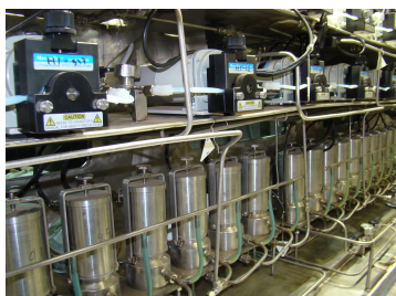
Figure 2 – ETsR-33 Extractors and Related Dosing Equipment
