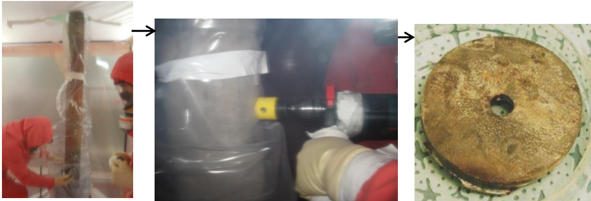
FIG. 6. Sampling in nuclear suit in the work airlock, example of a sample before decontamination (sample #GTEMP-CPML0373-02, red dots, FIG.3).
