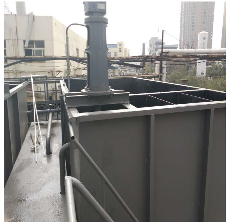
Flocculation and Sedimentation
